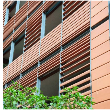
Horizontal louvres applied on a residential building - Lyon (France) Photo: S. Croce
