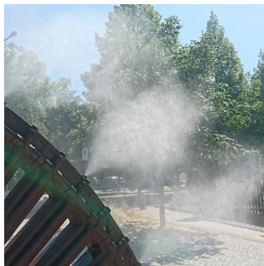
Mist spraying system - Prague (Czech Republic) Photo: S. Croce
