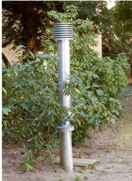
Figure 67: Ansitz Kofler . Inlet for the ventilation system pre-heating the air via the ground.
