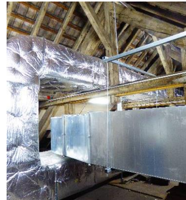
Figure 60: Elementary School "Cour de Lorraine", dual flow units in the attic
