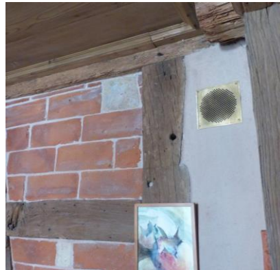
Figure 59: Timber-framed house in Alsace, supply air invisible between joists
