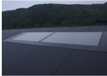
Figure 62: Integration of solar thermal panels in the roof of Doragno Castle .
