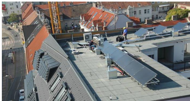
Figure 63: Mariahilferstrasse . Solar thermal installation on the roof.
