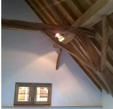
Figure 16: Half timberframed house in Alken, old roof truss with some new elements
