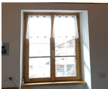
Figure 30: Mairhof . All windows were replaced.
