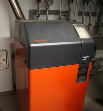
Figure 70: Rainhof . Biomass boiler that together with a biogas boiler produces heat and hot water.
