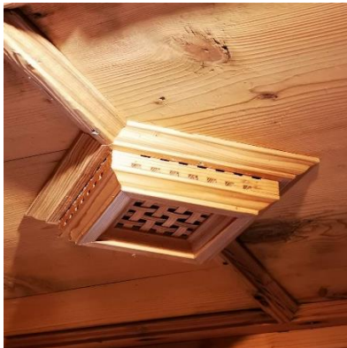
Figure 58: farm house Trins, ventilation ducts
