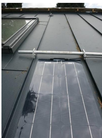
Figure 65: Villa Castelli . PV-panels integrated in the roof.
